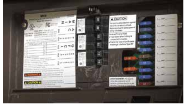
Typical 30 Amp circuit breaker and fuse panel. Note circuit and device labels.
