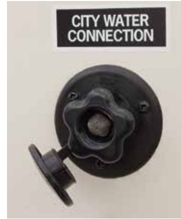
Typical city water fill connection
