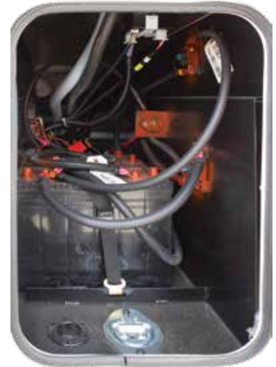
Typical Class A motorhome auxiliary (house) battery compartment
