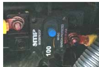
Typical Inverter Circuit Breaker located in the battery compartment.
