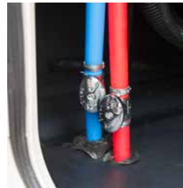
Typical low-point drain valves
