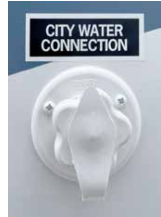
Typical city water fill connection
