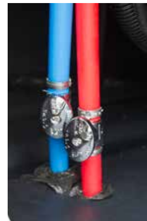
Typical low-point drain valves
