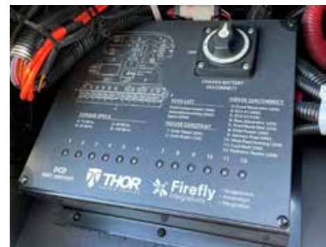
Master battery switch located on 12-volt circuit breaker panel.
