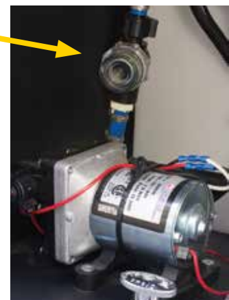
Water pump strainer
