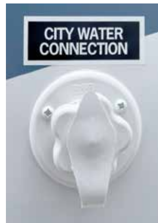
Typical city water fill connection
