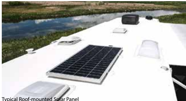
Typical Roof-mounted Solar Panel
