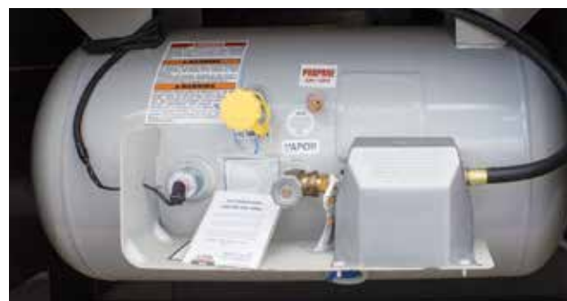
Typical permanently-installed RV propane tank with regulator
