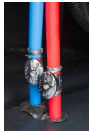
Typical low-point drain valves
