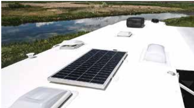
Typical Roof-mounted Solar Panel
